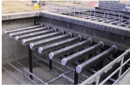
b. Aerobic MBBR with horizontally mounted cylindrical bar sieves
