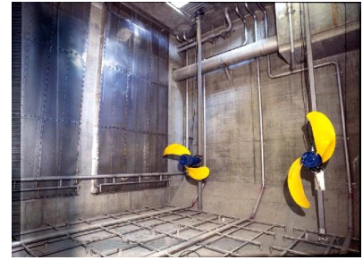
c. Anoxic MBBR with horizontally mounted shaft mixers and rectangular sieves
